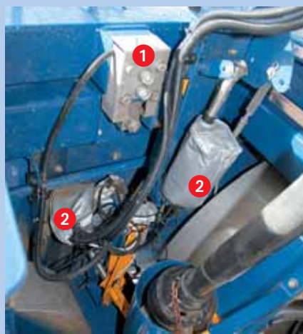
View from below: the weighing cell (1) is screwed on better than before. The laying of cables could be more elegant. Dust protection bags (2) protect the three servo motors.
